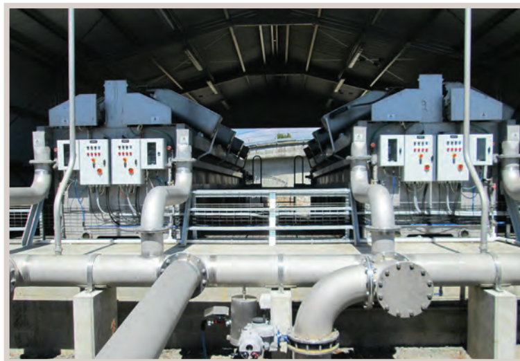
FILTRATION SYSTEM - TE KUITI WASTEWATER TREATMENT PLANT
