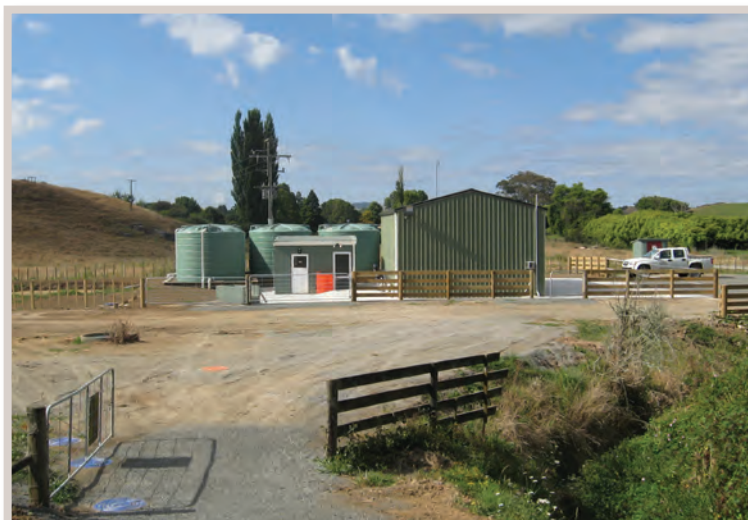
PIOPIO WATER TREATMENT PLANT
