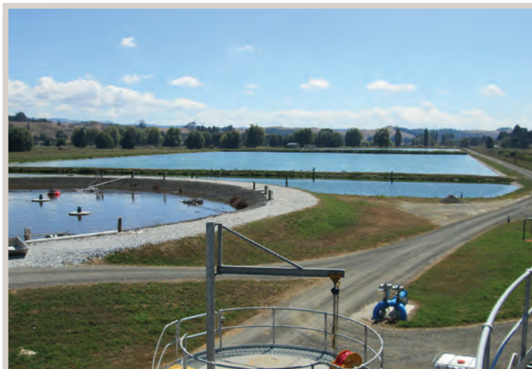
OVERVIEW - TE KUITI WASTE WATER TREATMENT PLANT
